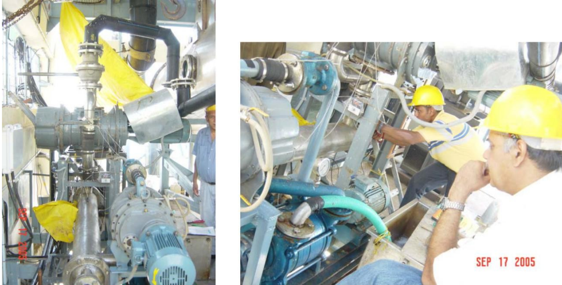
Fig 3 & 4: Everest Vacuum System for LTTD installed at Kavaratti (Lakshadweep)
